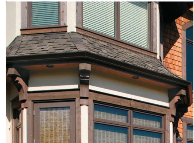
Ensure that all eaves are closed in and screen all vents and soffits.
