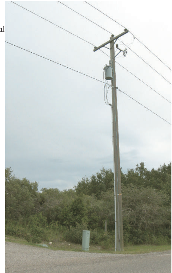
Ensure power lines are clear of all vegetation.
