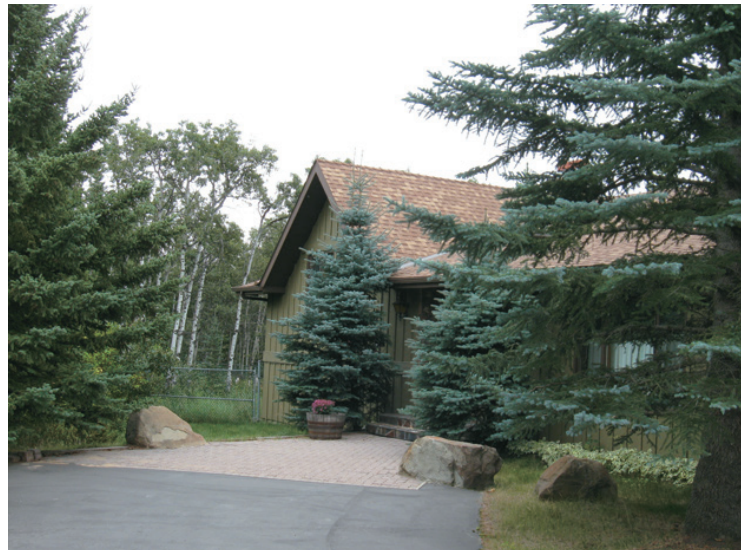
Coniferous trees located directly next to a building can allow wildfire to come in close or direct contact with a building.
