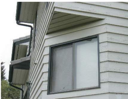
Wooden siding offers very little fire resistance.
