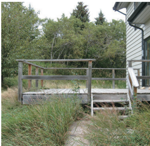
Flammable material under and around decks can pose a fire hazard.
